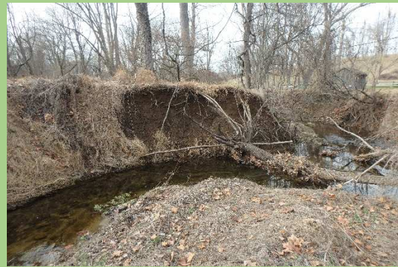
Pre-Restoration Sediment Deposits and Eroded Streambank
