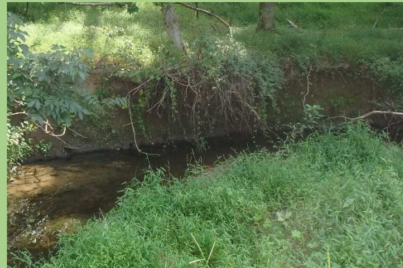
Pre-Restoration Sediment Deposits and Eroded Streambank
